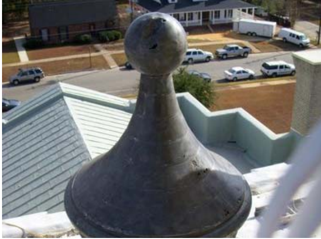
STRIPPED AND PITTED FINIAL
