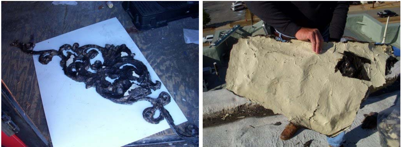
FOLIATE ORNAMENT MIDWAY IN RESTORATION AND, BEFORE, ENCRUSTED IN TAR AND PAINT
